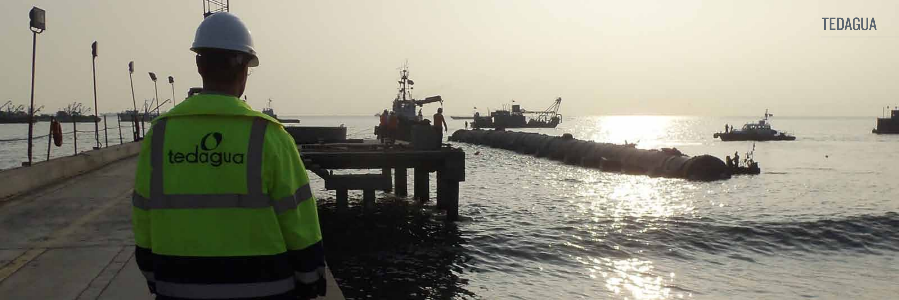
Installation of the submarine infall of the WWTP of Taboada (Lima, Peru)
