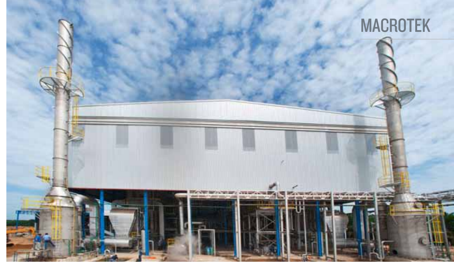
Biomass boiler exhaust MVA venturi scrubbers and stacks for biofuel power plant in Thailand
