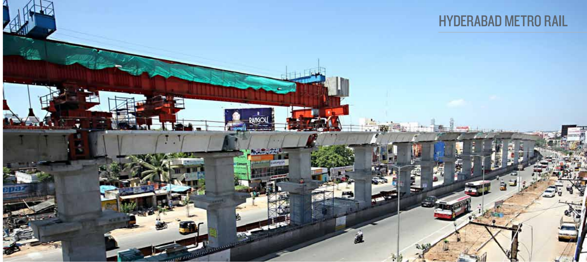
Launching Girder – State of the art construction equipment used to build elevated viaducts of Hyderabad Metro Rail
