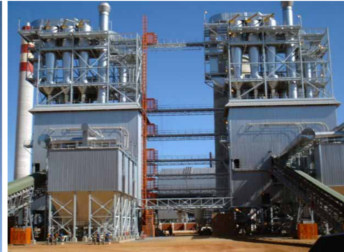
Platinum concentrate – flash dryer – Anglo American Platinum
