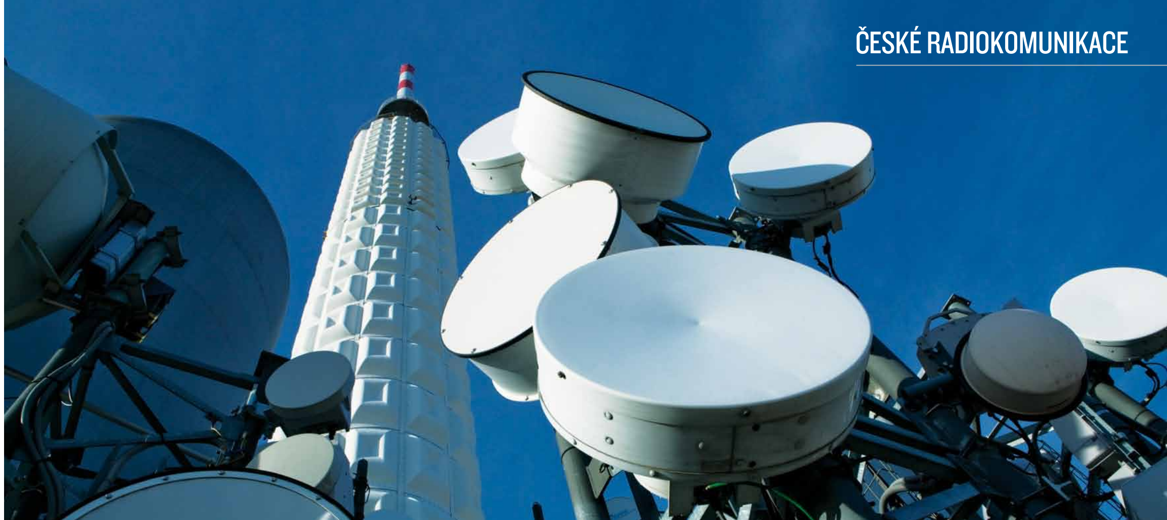
Microwave radio technology (at Prague tower)
