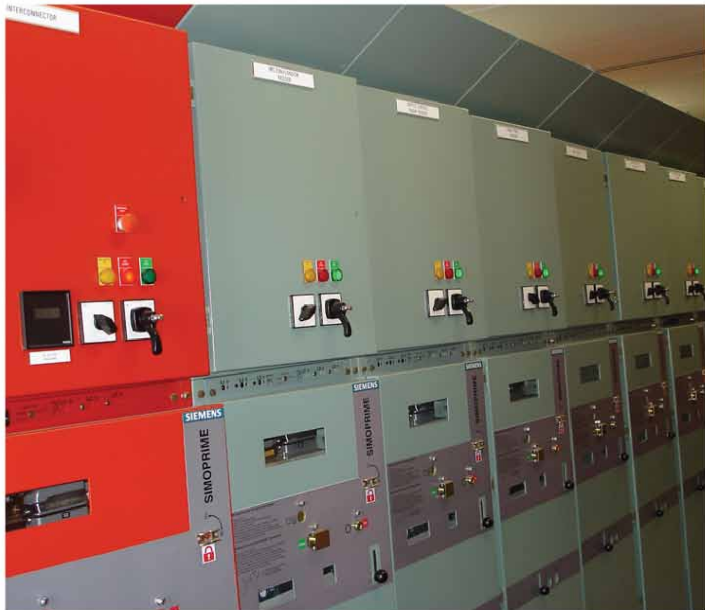
Installed modular SIMOPRIME switchgear - City Power's Alexandra Substation.
