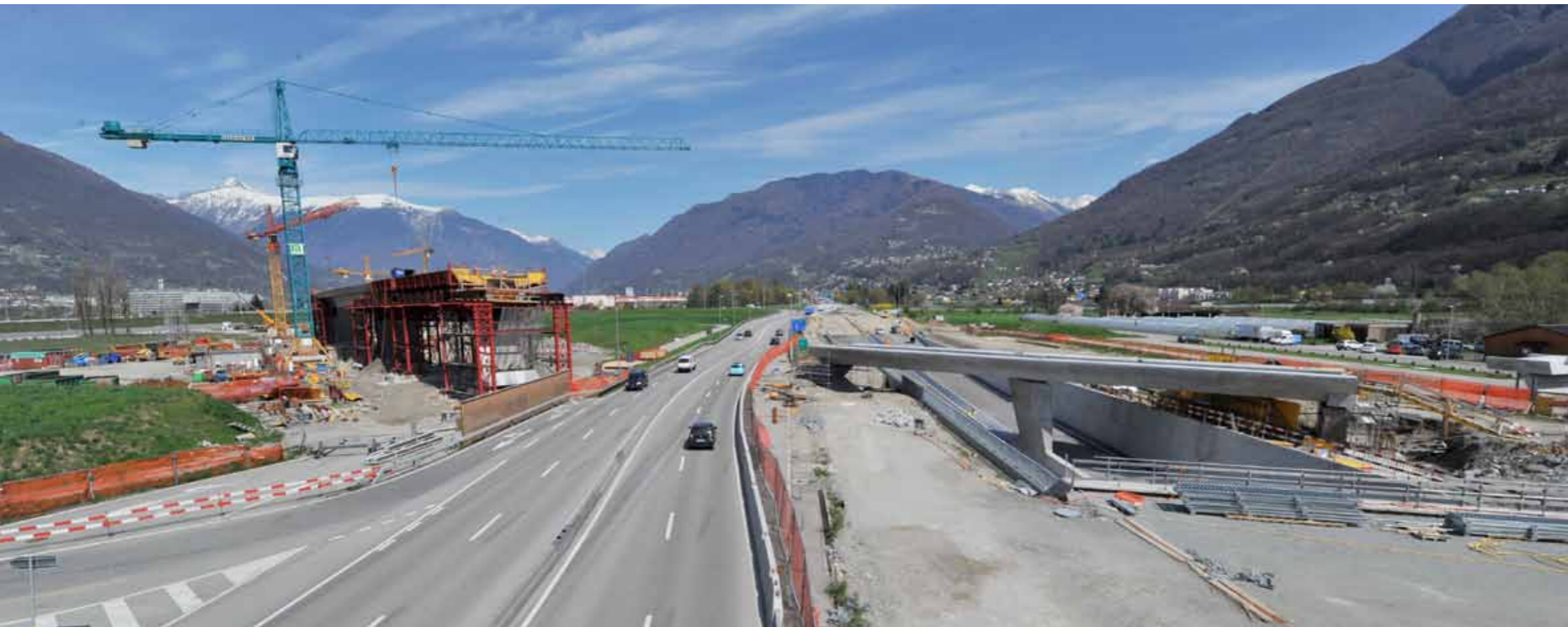
Work in progress at Camorino, north of the north portal of the Ceneri Base Tunnel, includes the Lugano-Bellinzona viaduct and the new underpass of the cantonal road
