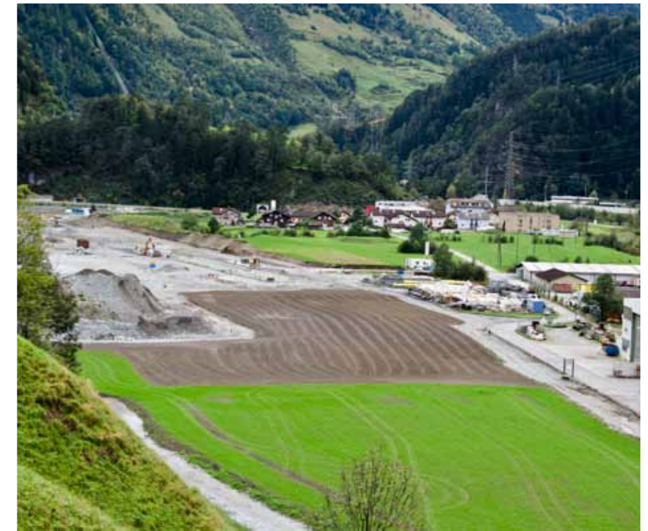
The Amsteg installations site has been removed and is now being renatured
