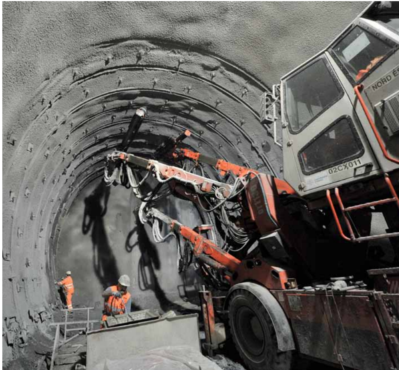
In the Ceneri Base Tunnel at Sigrino, progress continues on four drives
