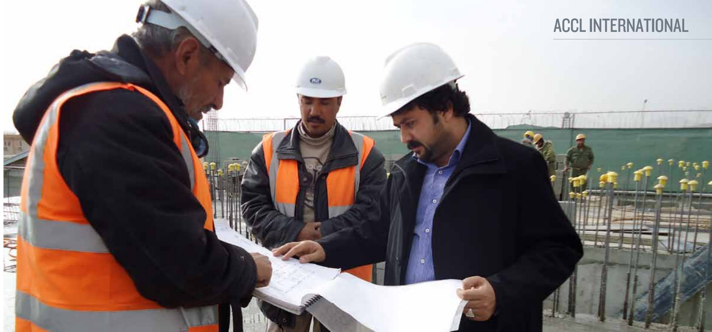
Company President, Habibullah Pirzada reviews the construction plans at Bagram, just outside of Kabul
