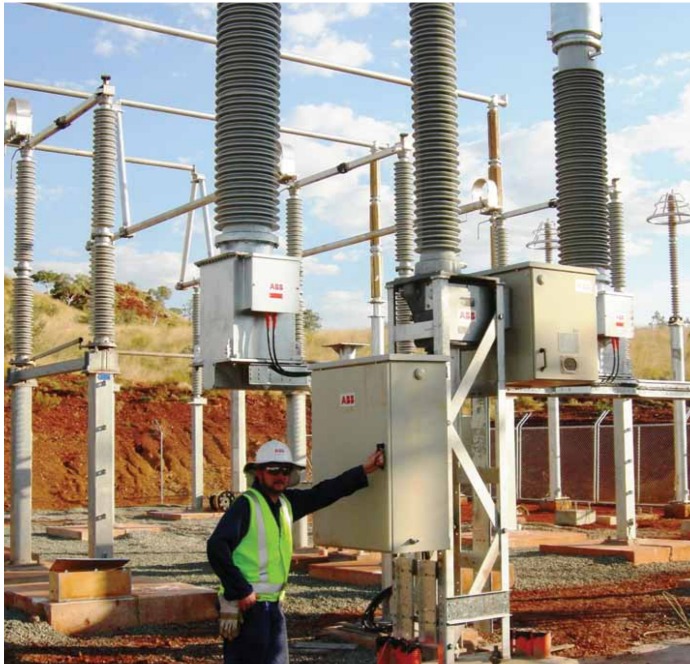
ABB substation at Rio Tinto Pilbara
