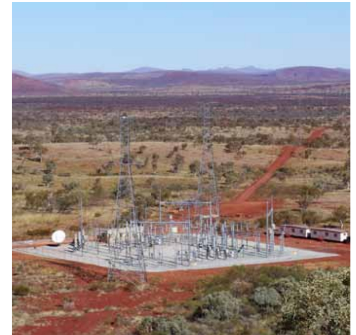
Juna Downs substation
