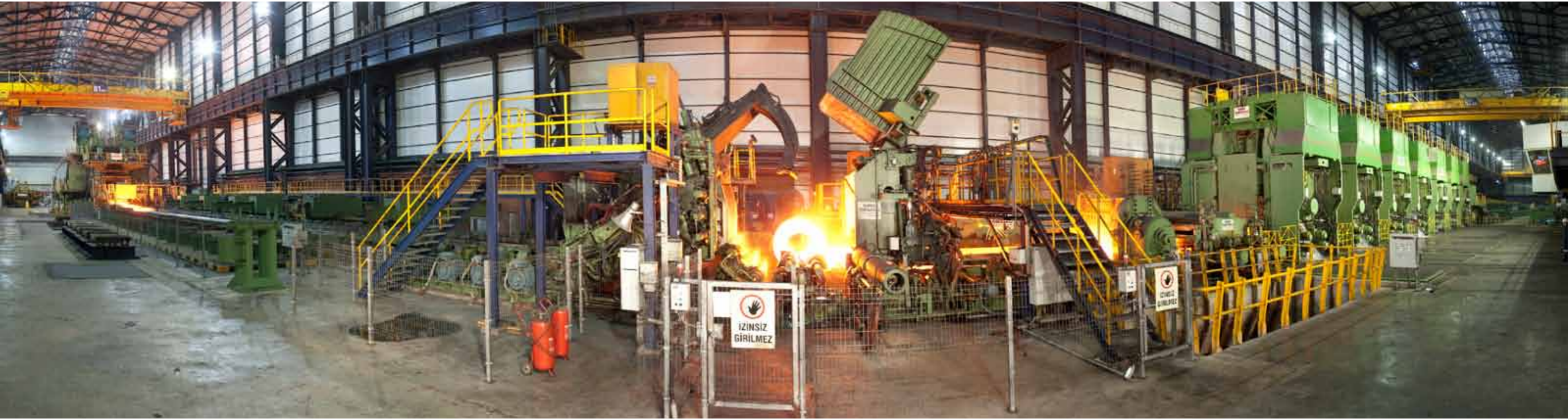
Panoramic view of the entire line
